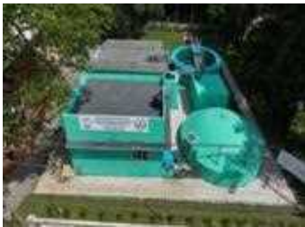
360 KLD STP at General Hospital, Thrissur
